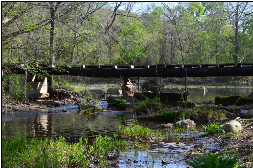
Illustration 12. Bridge propped up by stones over creek. Photo courtesy of Beth Ebbing.
